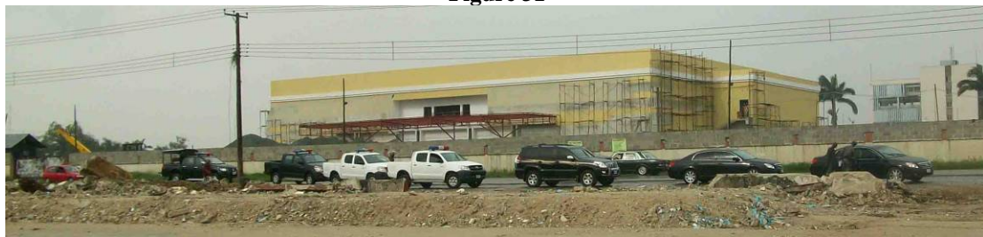
Silverbird Showtime under construction (12 March 2009); in the foreground, the rubble of buildings demolished (10-13 February 2009) to make way for a parking area © J. Falade
