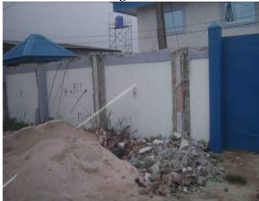
Partly demolished “illegal structures” that were erected beyond a plot boundary in GRA © R. Precht
