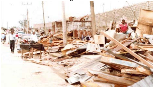
Demolished shops and houses along the lower part of Abonnema Wharf Road (September 2008) © NUTN
