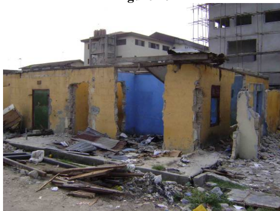
Legal structures in Nanka Street, demolished to make way for construction of a hospital (in the background) © R. Precht
