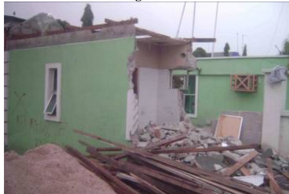
A wall that had encroached on the road reserve in GRA is marked for demolition © R. Precht
