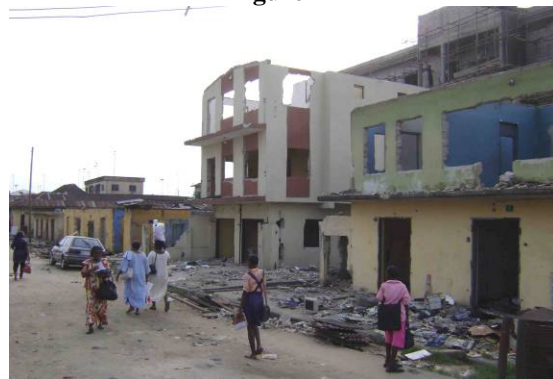
Demolished legal structures in Nanka Street; New Niger Hospital (under construction) in the background © R. Precht
