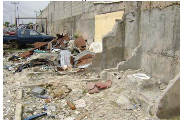
The toilet bowls are evidence that the demolished structures along the lower part of Abonnema Wharf Road had been much more than just temporary kiosks © R. Precht
